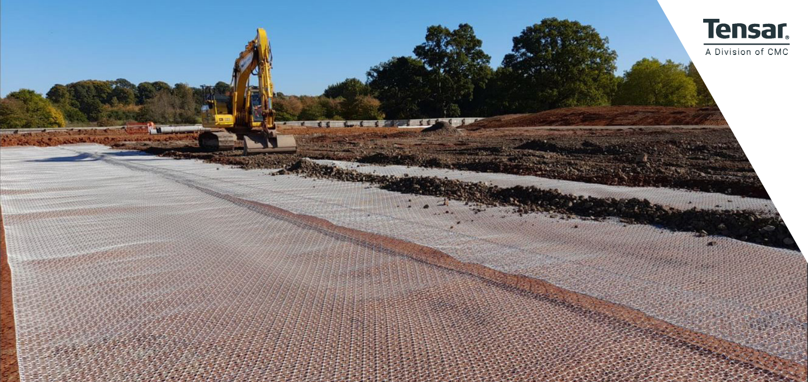
Installation of Tensor InterAx geogrid helped to save time, cost and carbon on the site's working platform
