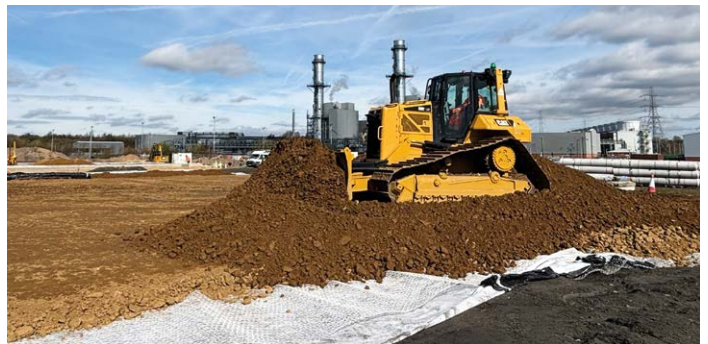
➤ Cryogenic Energy Storage Facility BESS
