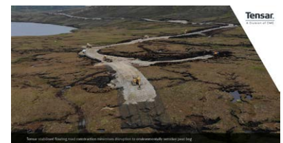
Roads and Platforms № 476
